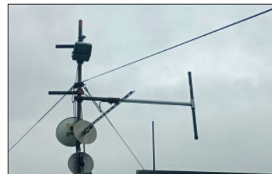
Antenna for Kaikoura 690 installed on mast
