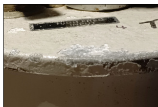
Surface corrosion on top of filters
