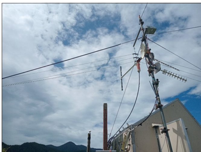
Figure 6, Hut and antenna array
